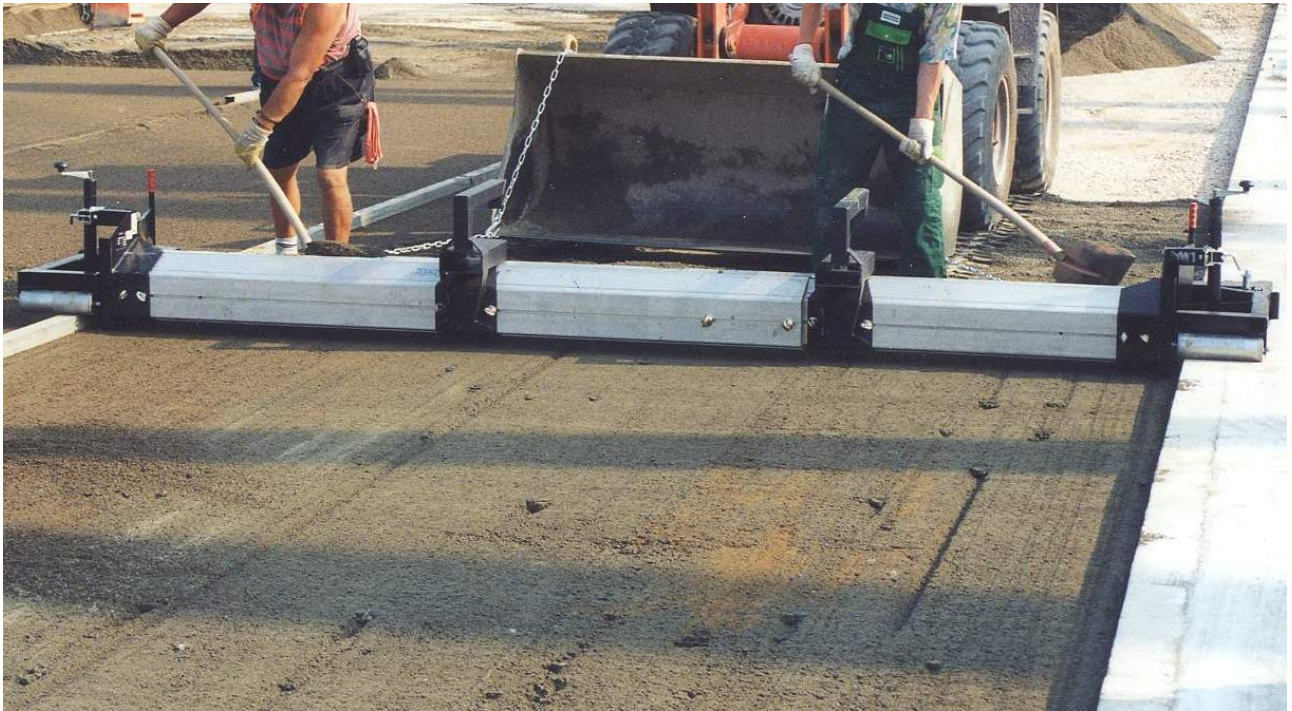
TAK without TAK-DP Figure 2
